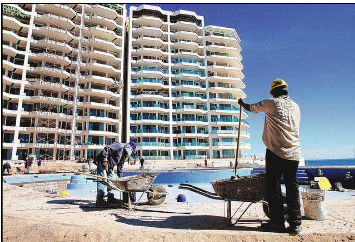
Construction workers prepare concrete for one of four pools outside the Esmeralda resort condominium on Puerto Peñasco's Sandy Beach. Photos By Greg Bryan / arizona daily star
